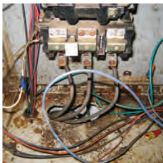
Corrosion leads to premature component failure
